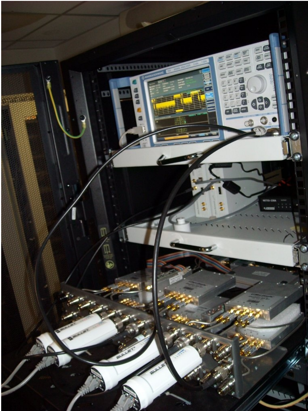
Figure 39: RF network installed in rack
