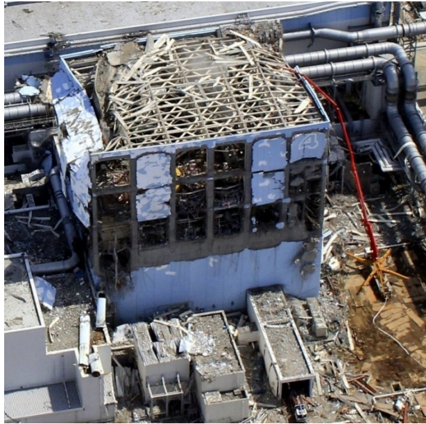
Figure 37. The destroyed building of reactor No. 4 of the Fukushima Daiichi nuclear power plant [87].
